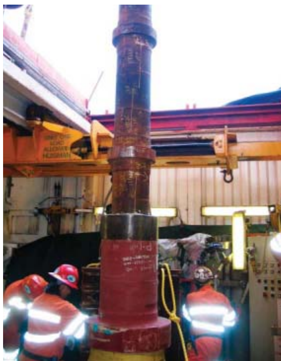
Bulk head installation: Inner pipe is pulled out to proper inner pipe tension.
