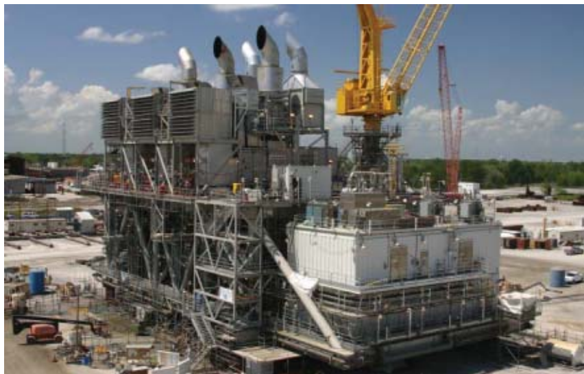
J. Ray McDermott constructed three modules for the Atlantis topsides. The production and compression modules are each approximately 5,000 tons, and the power generation module (pictured) is approximately 4,000 tons in weight.
