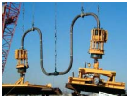
Installation of the Test Jumper between the PLET & WYE sled for BP Mardi Gras project.
